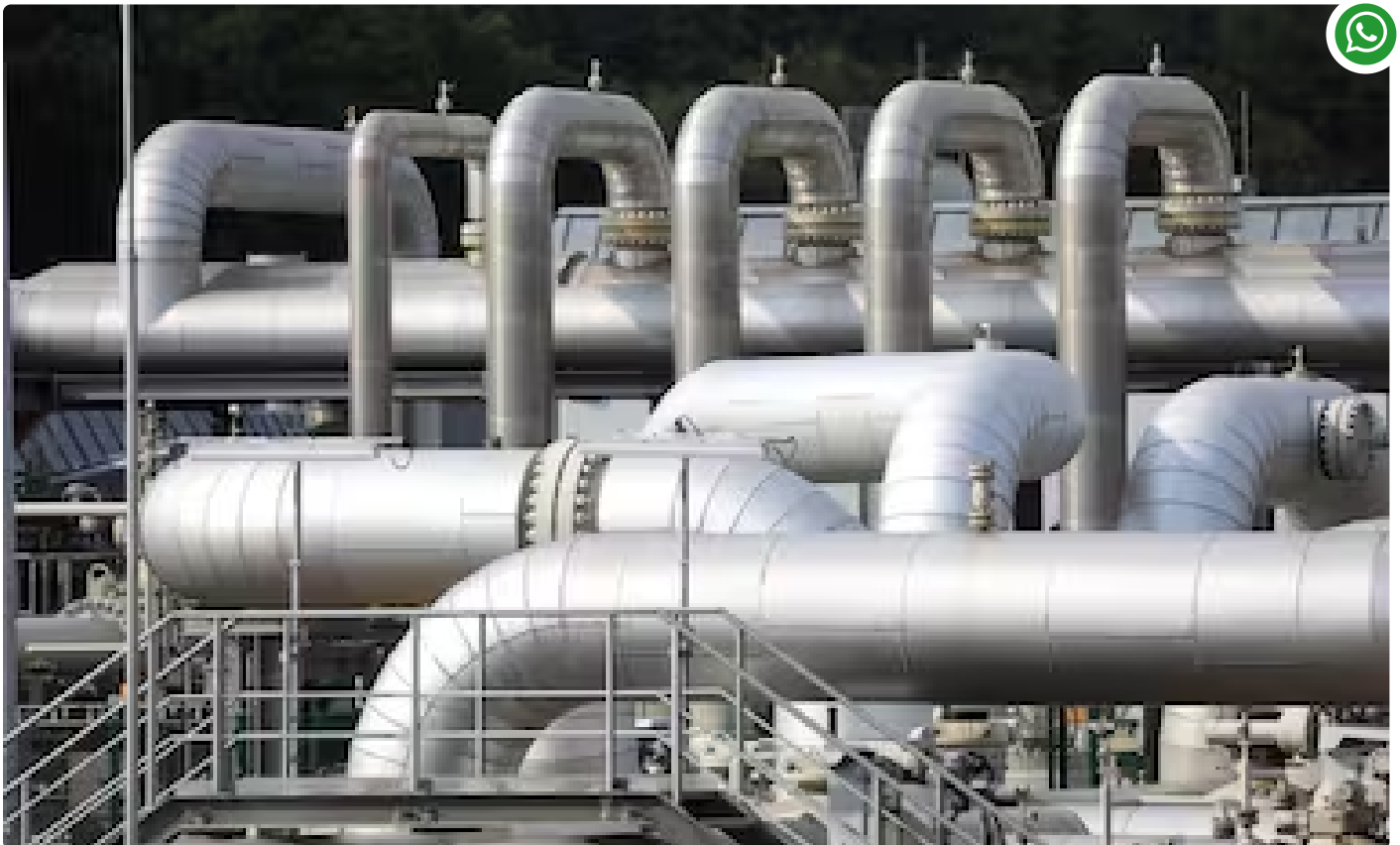
Pipework at the natural gas storage facility operated by Astora GmbH & Co KG, one of the largest in Western Europe. Photographer: Krisztian Bocsi/Bloomberg
